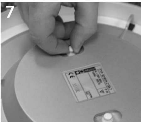
7 Pull cover-plate buttons on back of fixture and remove coverplate.
