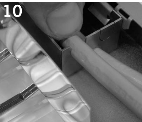
10 Seat cord into void left from cord removal. NOTE: Cord must be properly seated for replacement of splice compartment cover.
