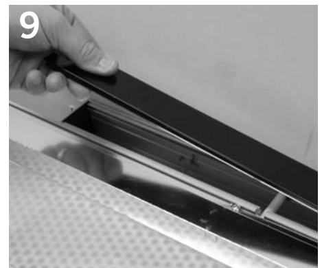
9 Replace plastic coverplate. Install lamps per relamp label.
